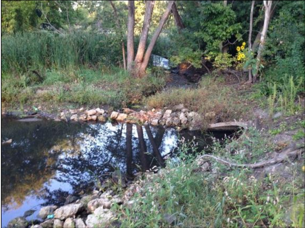
Bassett Creek Side Channel and Trail Work (work paid for by MPRB and city of Minneapolis) – AFTER
