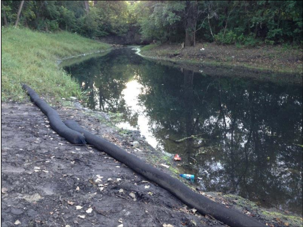
Bassett Creek Side Channel and Trail Work (work paid for by MPRB and city of Minneapolis) – AFTER
