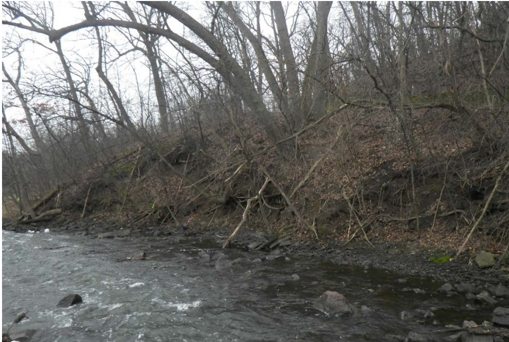
Photo 5. Site 5. Moderate erosion on steep bank
