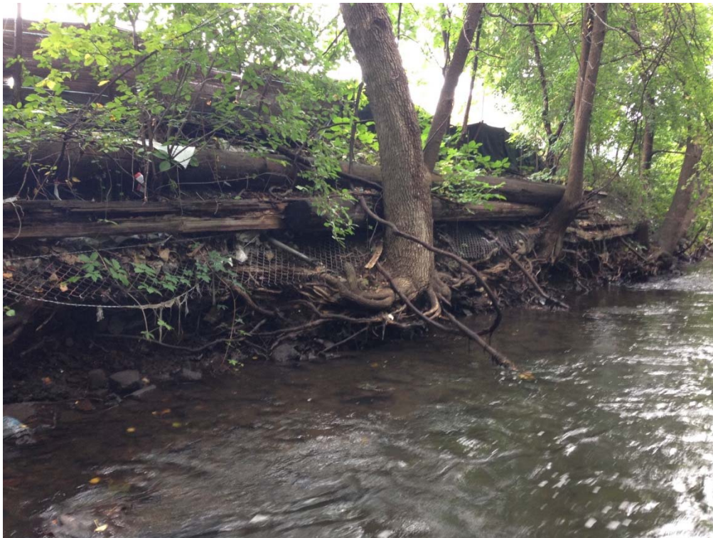
Photo 6. Site 6. Steep eroding bank
