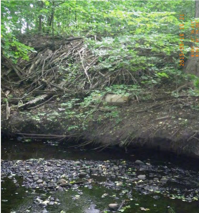
Photo 13: Debris (hot water heater, plastic, wood) in bank of creek east of Fernbrook Lane
