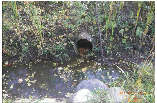
Photo 10: Wetland 4 facing southeast. Culvert reveals one potential source of hydrology for Wetland 4.
