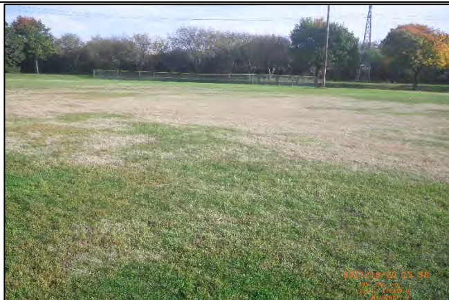
Photo 11: Area that occasionally becomes inundated after a rain event located southwest side of Bryn Mawr Meadow Park.
