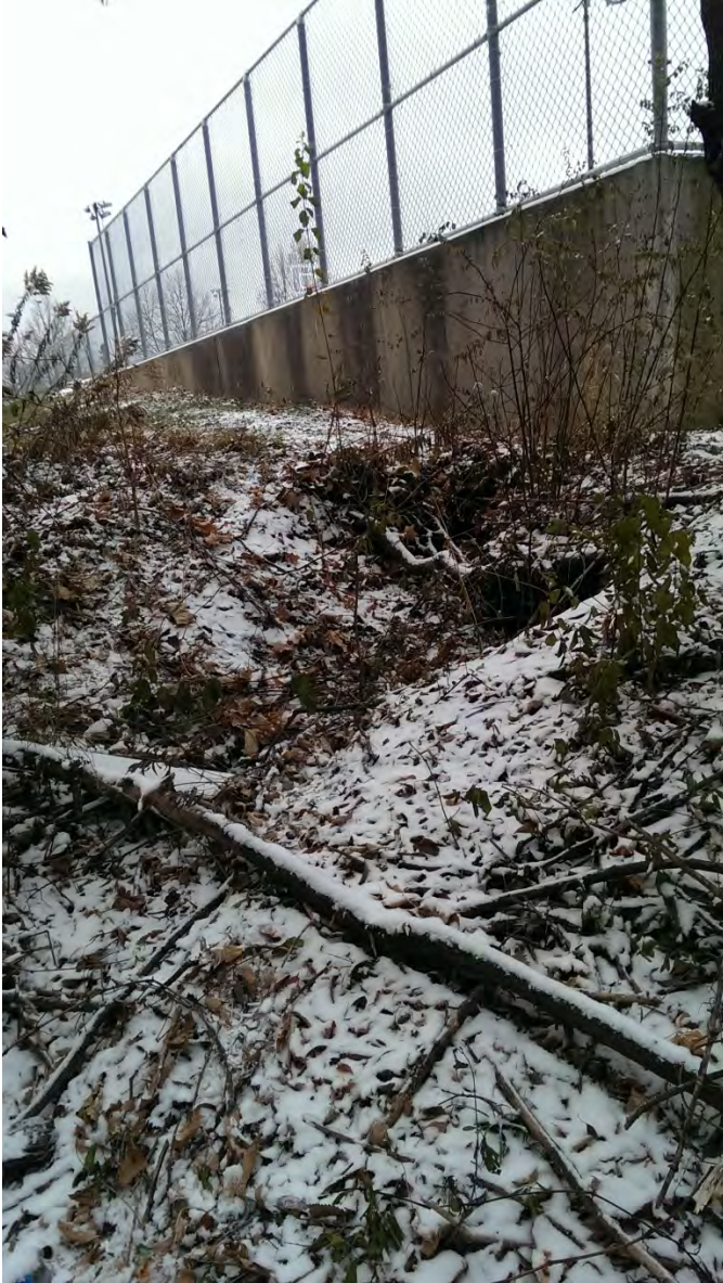
Figure 28 – Parkers Lake, Reach 1, slope erosion cause by recreation courts runoff
