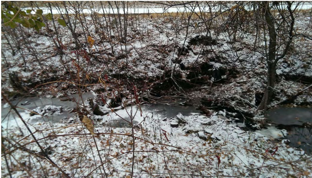
Figure 40 – Parkers Lake, Reach 2, bank scarp erosion
