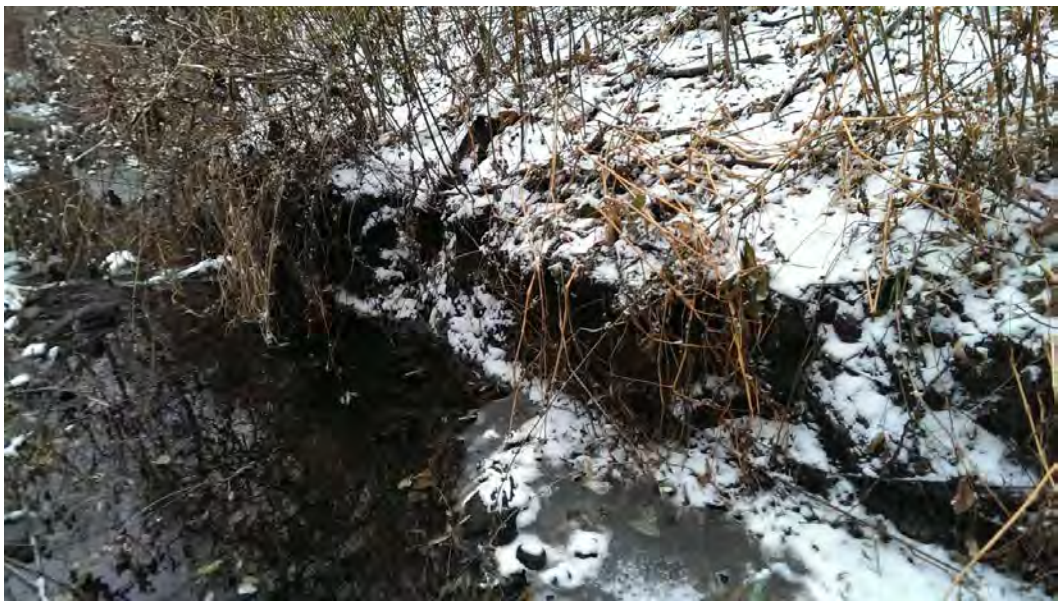
Figure 33 – Parkers Lake, Reach 1, undercut bank (zoomed in of previous figure)
