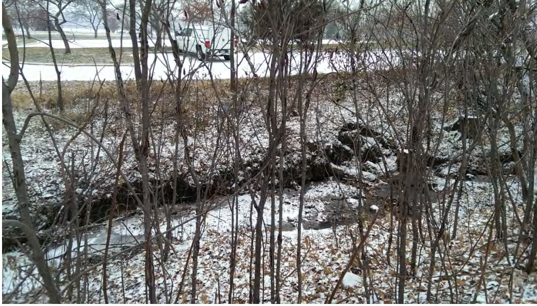
Figure 41 – Parkers Lake, Reach 2, bank erosion
