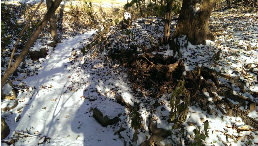
Figure 1 – Mt. Olivet, Reach 1, undercut bank erosion
