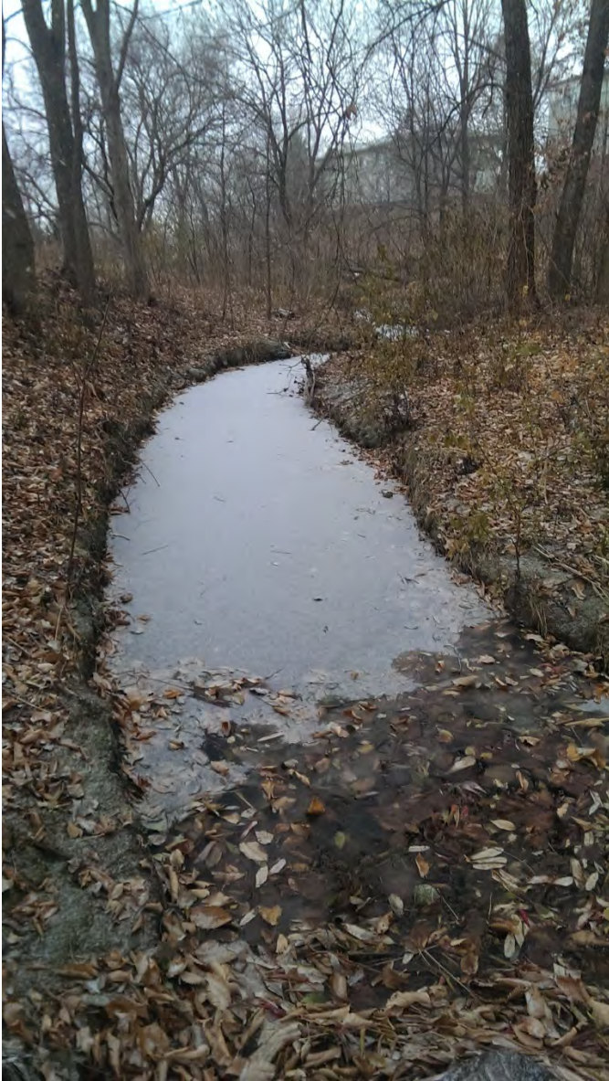
Figure 49 – Parkers Lake, Reach 2, bank erosion
