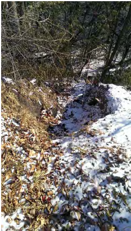
Figure 12 – Mt. Olivet, Reach 2, slope erosion from parking lot to the stream (view from above, same location as previous figure)
