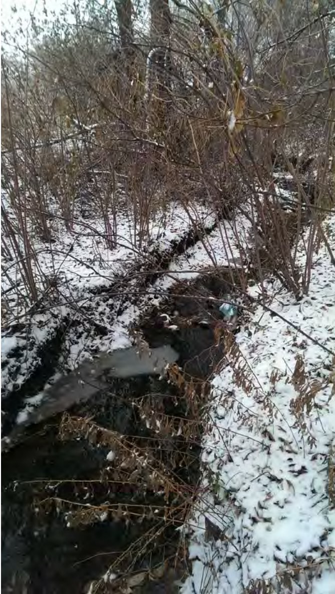
Figure 36 – Parkers Lake, Reach 1, bank erosion
