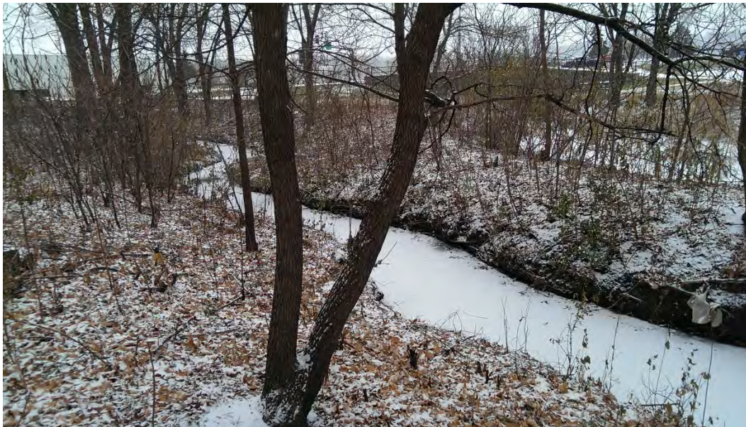
Figure 44 – Parkers Lake, Reach 2, undercut bank and bank erosion
