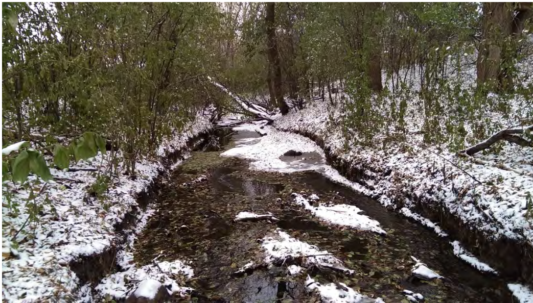
Figure 22 – Parkers Lake, Reach 1, bank erosion
