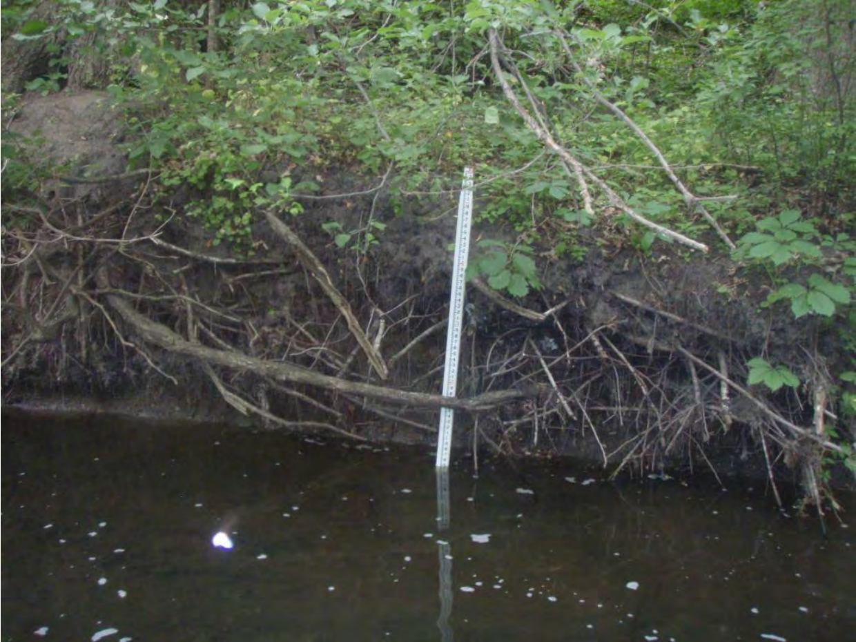
Photo 20. Site 18. Moderate erosion with undercut trees.
