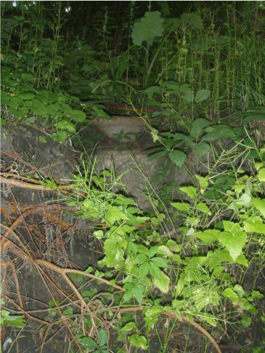
Photo 12. Site 10. Manhole in need of additional support and protection.
