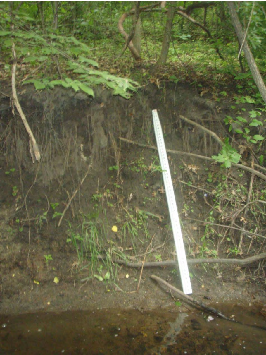
Photo 15. Site 13. Scarp formation with severe erosion
