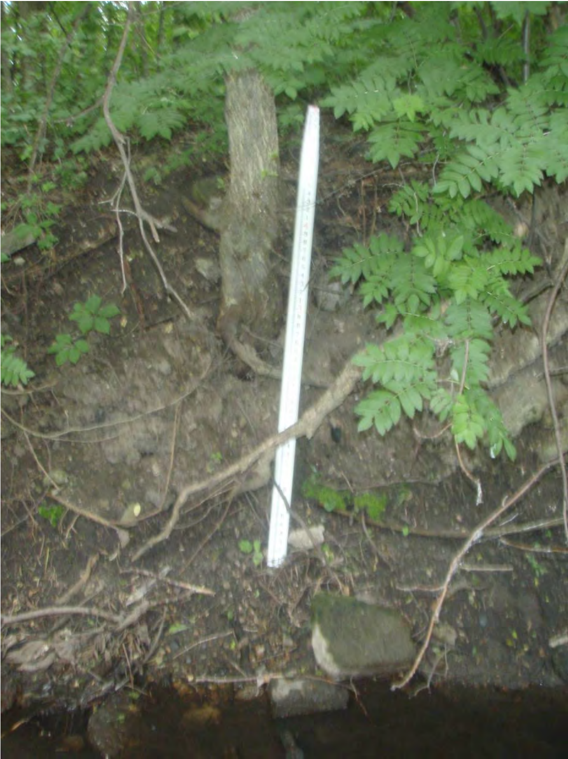
Photo 21. Site 19. Steep bank with erosion present.
