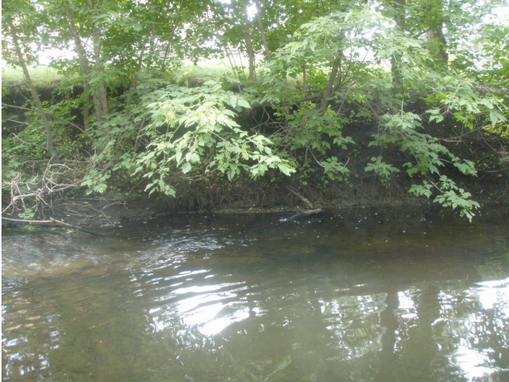
Photo 15. Site 15. Minor bank erosion.
