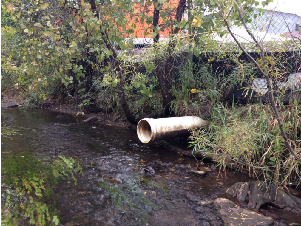
Photo 10. Site 10. Protruding Culvert
