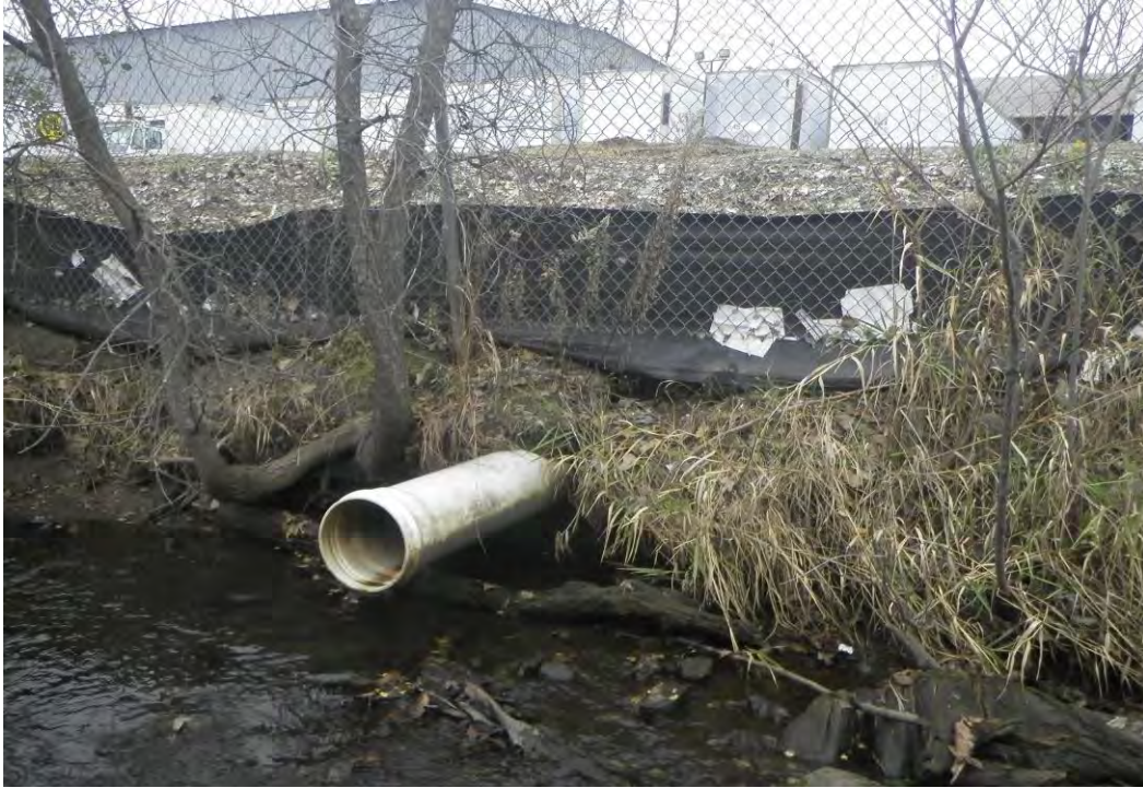
Photo 11: Example of discharge pipe
