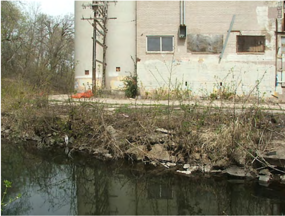
Photo 23: Fruen Mill Side of Creek showing cement debris and rip rap attempts at controlling erosion.
