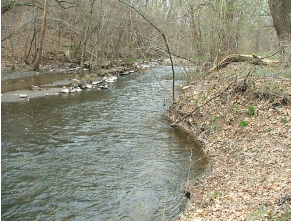
Photo 3: Eroded Retaining Wall “Rapids”.
