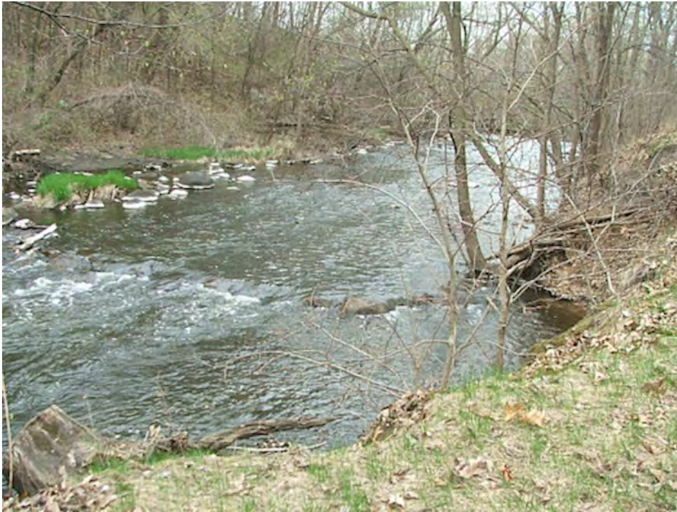
Photo 6: Eroded Retaining Wall "Rapids".
