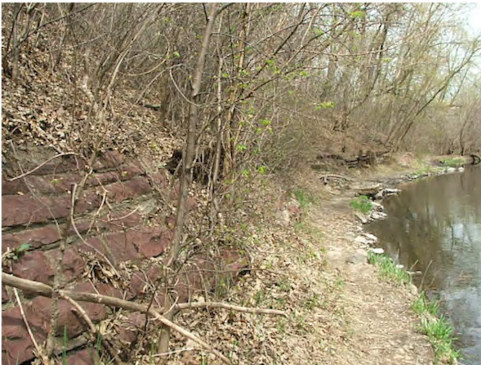
Photo 10: Bassett Creek Park Trail (note erosion).
