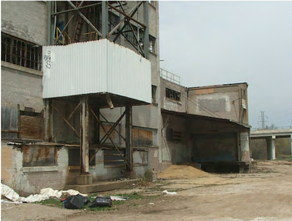
Photo 20: Deterioration and demolition of Fruen Mill.
