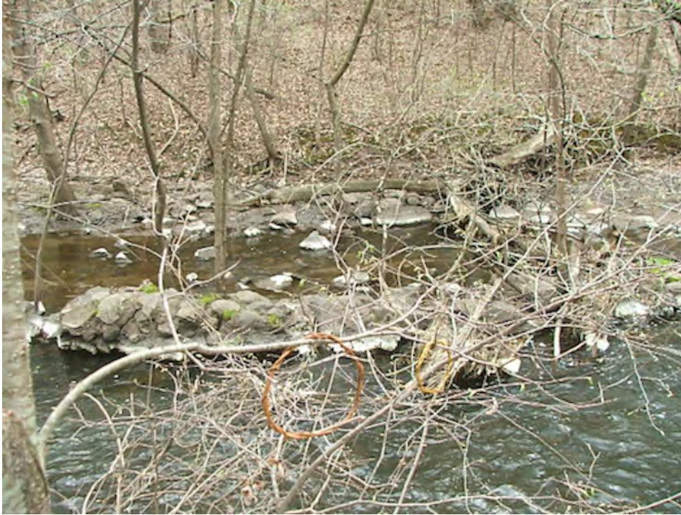
Photo 5: Eroded Retaining Wall "Rapids".
