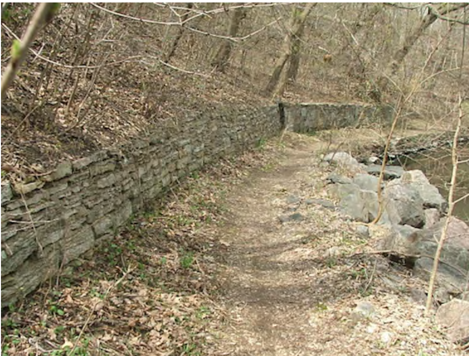
Photo 14: Bassett Creek Park Retaining Wall and Rip Rap along eroding park trail.
