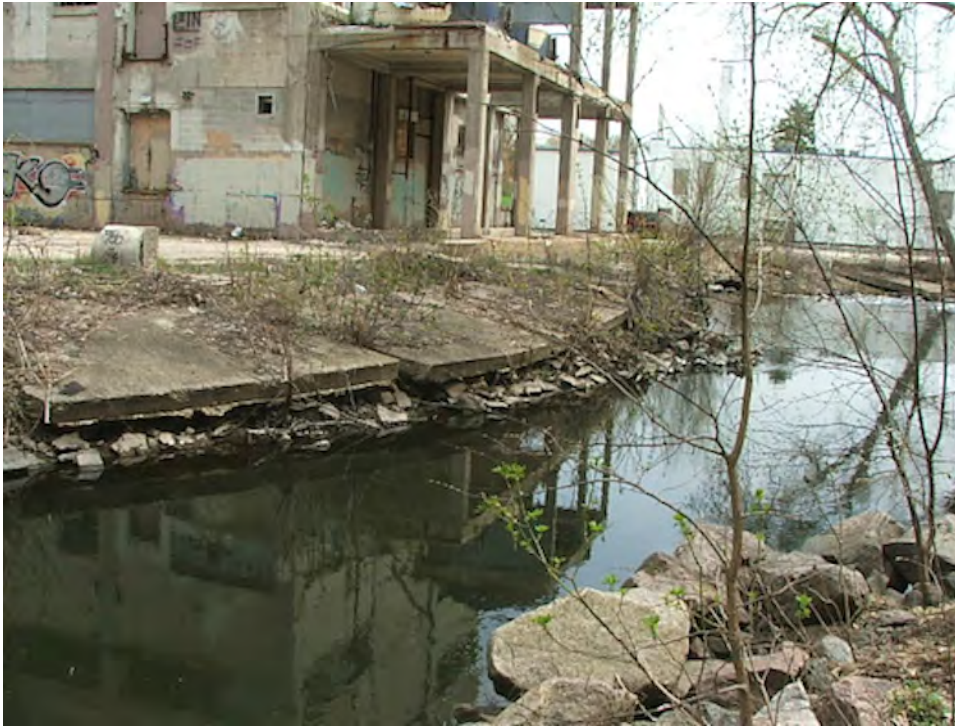
Photo 15: Fruen Mill and Bassett Creek (note slumping creek bank cement slabs).
