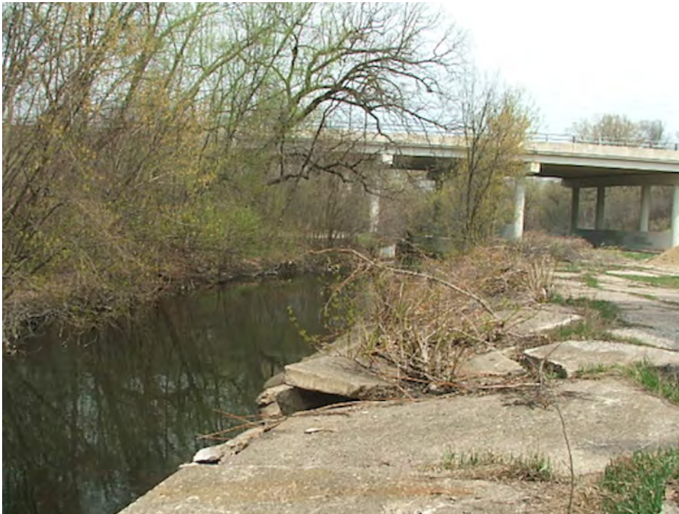
Photo 24: Deteriorating Concrete on Fruen Mill Side of Creek.
