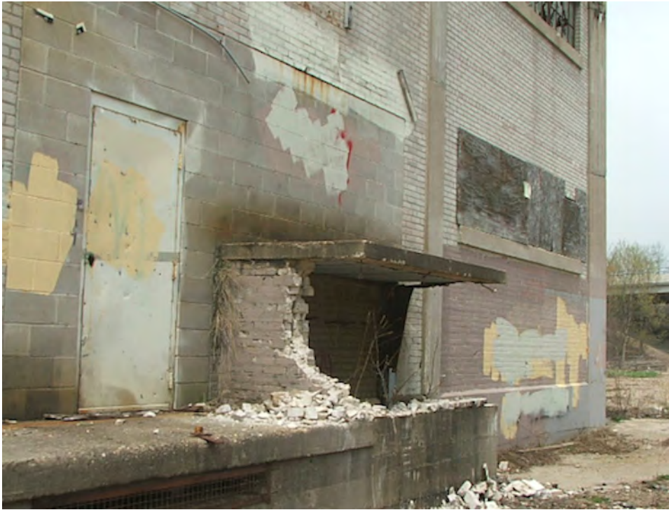
Photo 19: Deterioration and demolition of Fruen Mill.
