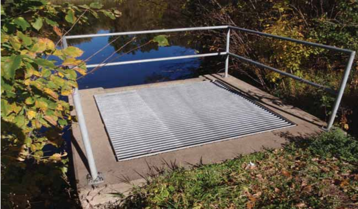
Detention Pond Outlet Structure (Crystal)
