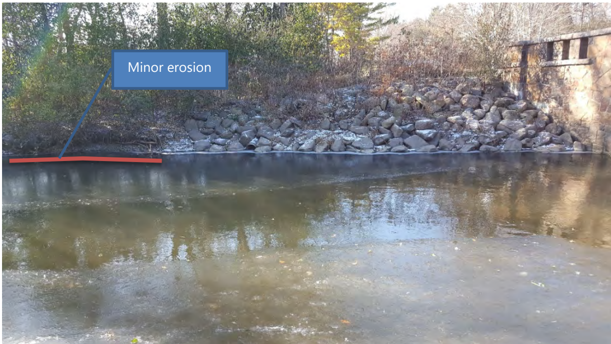
Figure 3-5 Erosion within right overbank of the channel downstream of the riprap (upstream of Lagoon E)
