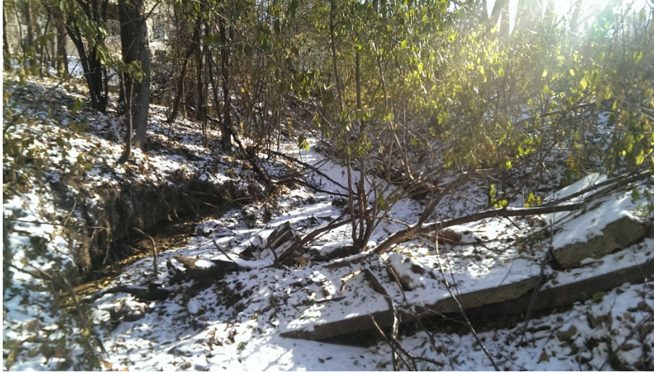
Figure 3-2 Mount Olivet Erosion Example (broken concrete causing stream to erode bank at left)
