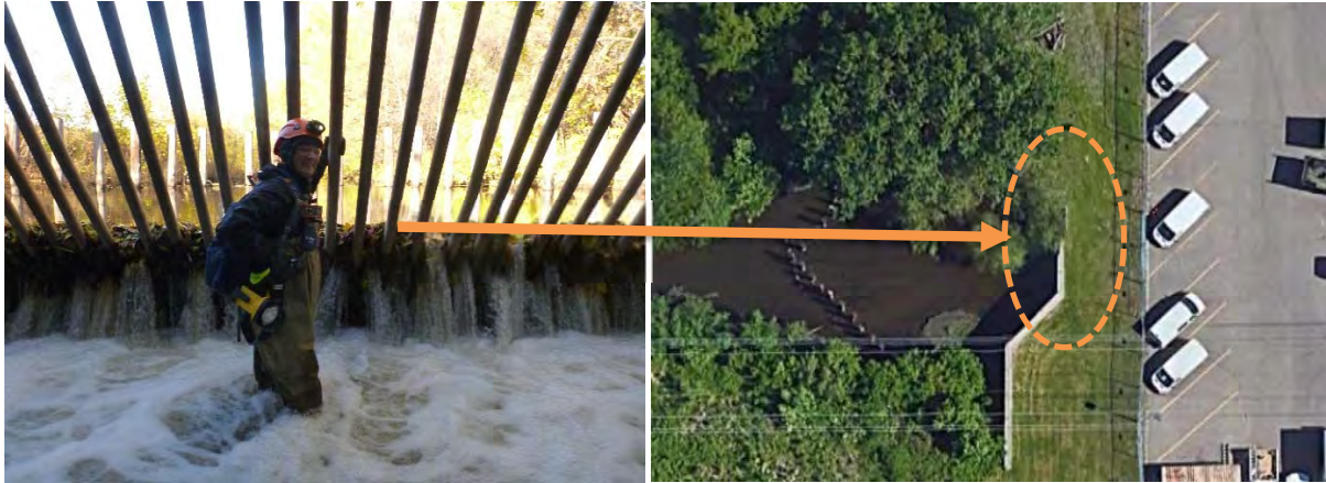
Figure 3-1 Trash Rack Debris
