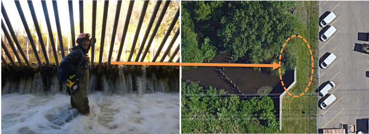
Figure 3-1 Trash Rack Debris
