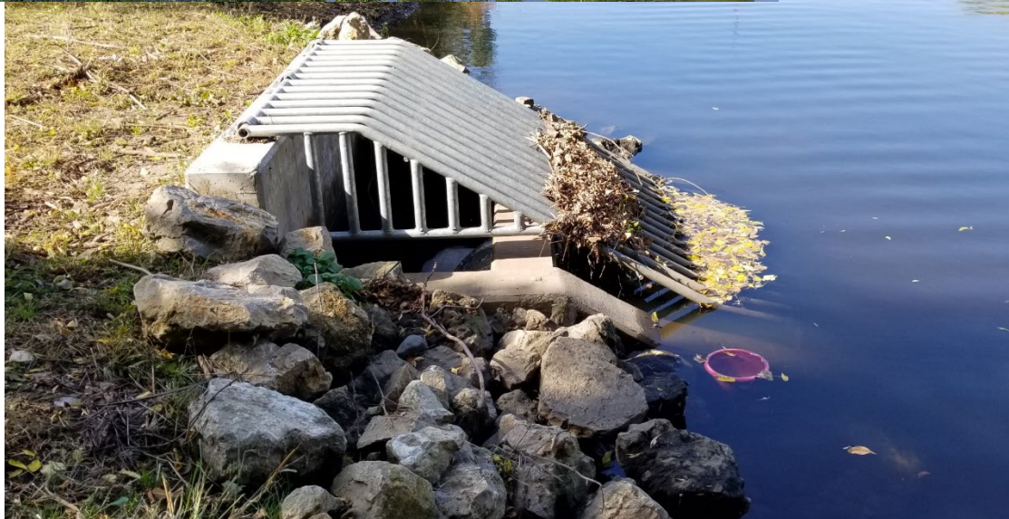
New outlet structure with trash rack and riprap
