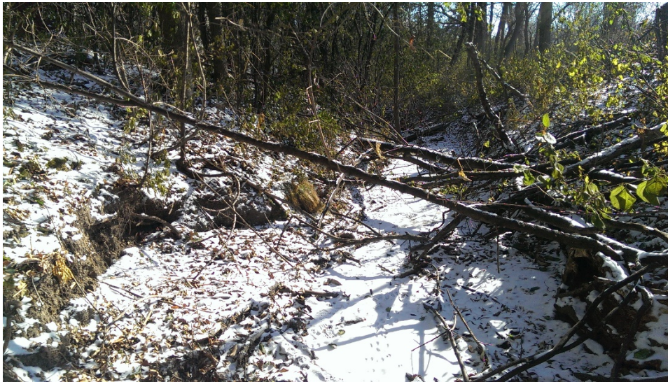
Figure 3-3 Mount Olivet Erosion Example (bank erosion)
