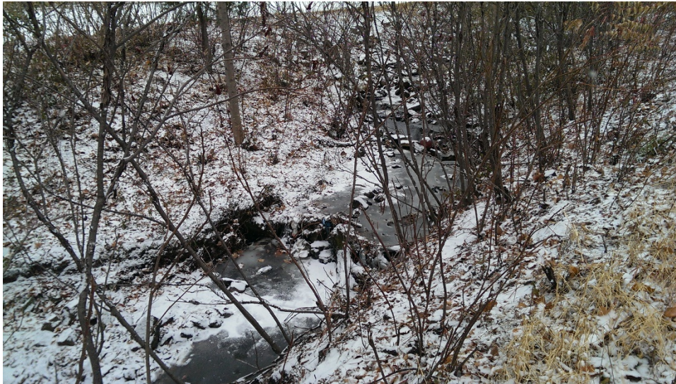
Figure 3-7 Parkers Lake Erosion Example
