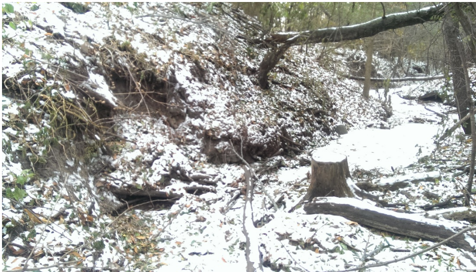
Figure 3-5 Mount Olivet Erosion Example 4 (bank erosion)
