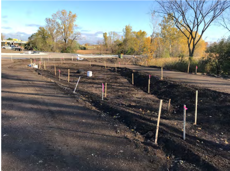
North Rain Garden – North View
