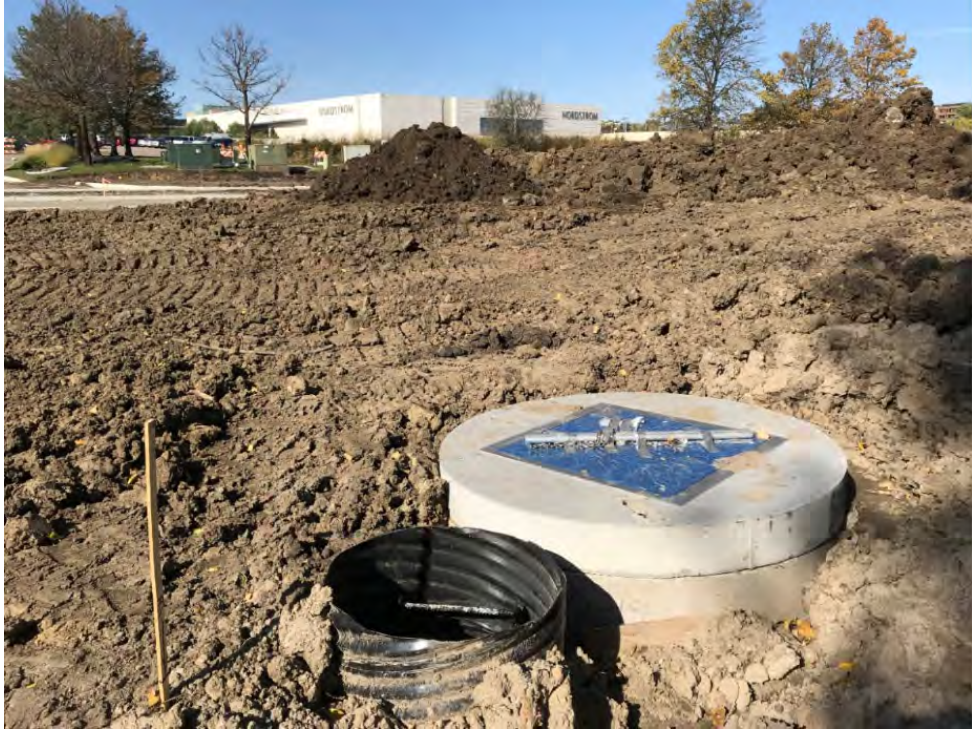
Storm Water Lift Station Access Structures at Crane Lake Park – West View
