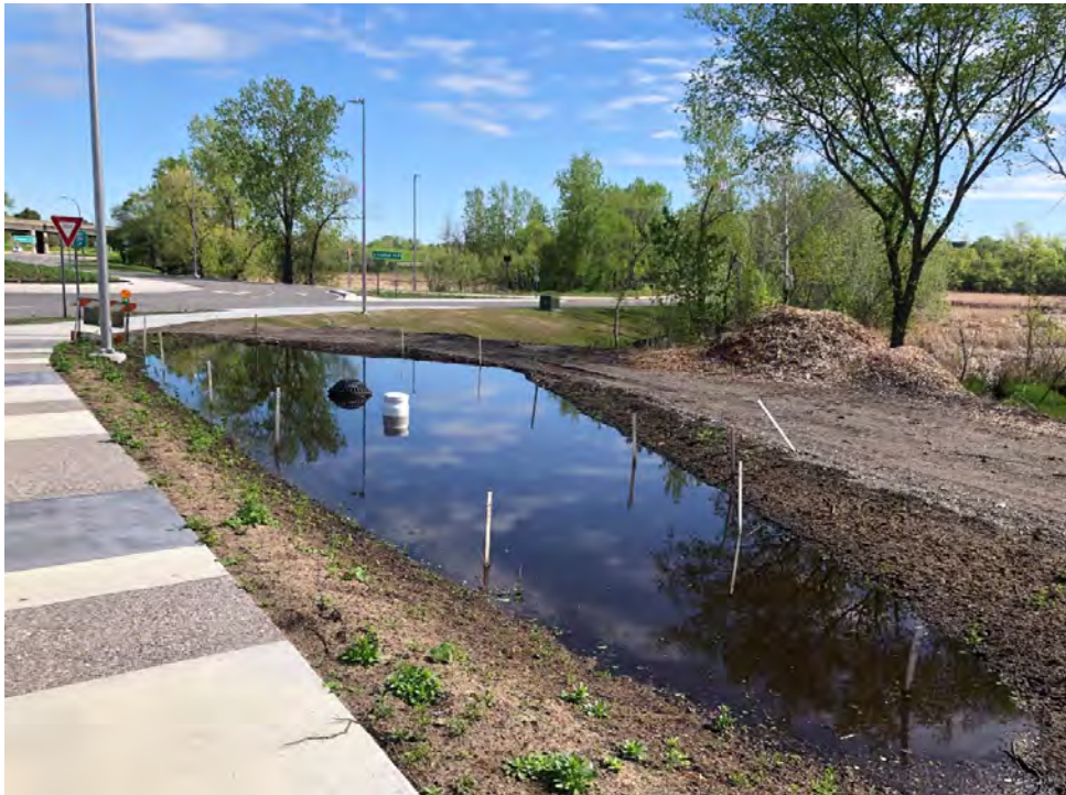
North Rain Garden (Valve Closed – Filtration Needed) – North View
