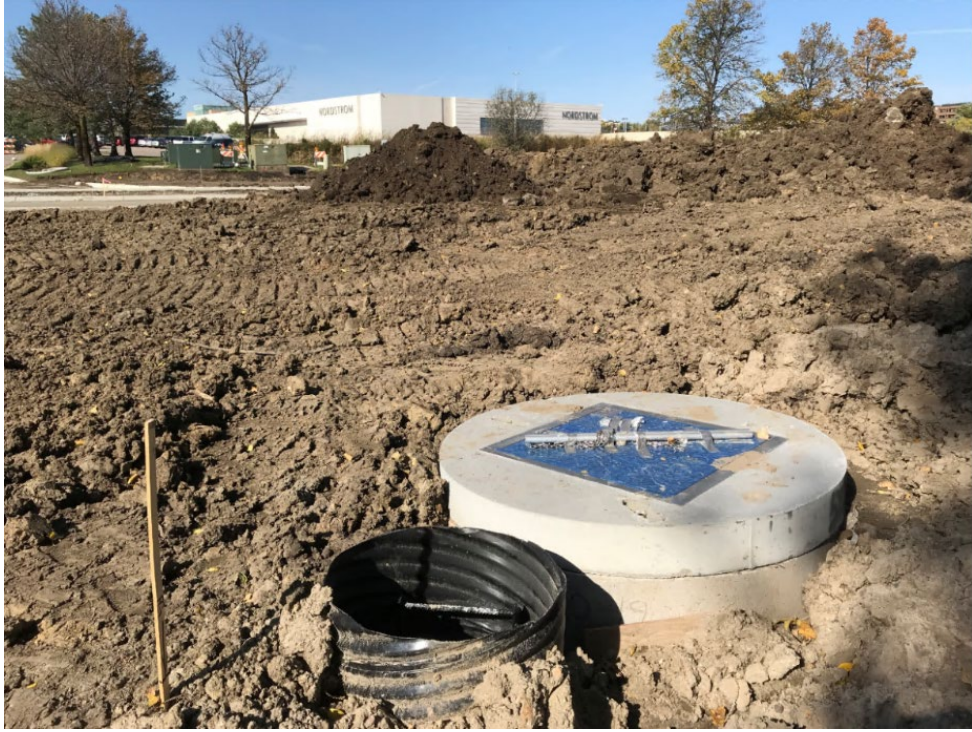
Storm Water Lift Station Access Structures at Crane Lake Park – West View
