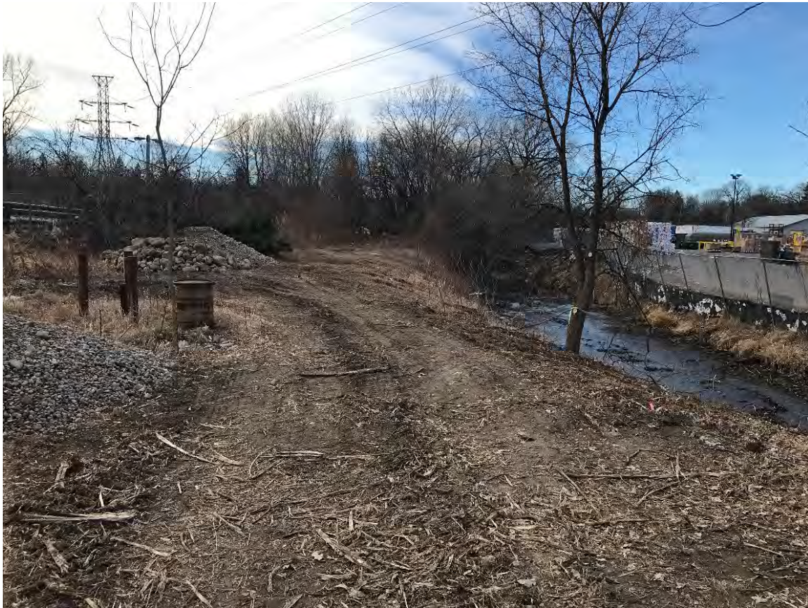
Reach 1: Southern bank following tree and shrub clearing. Drum disposed of at landfill (12/3/2020)
