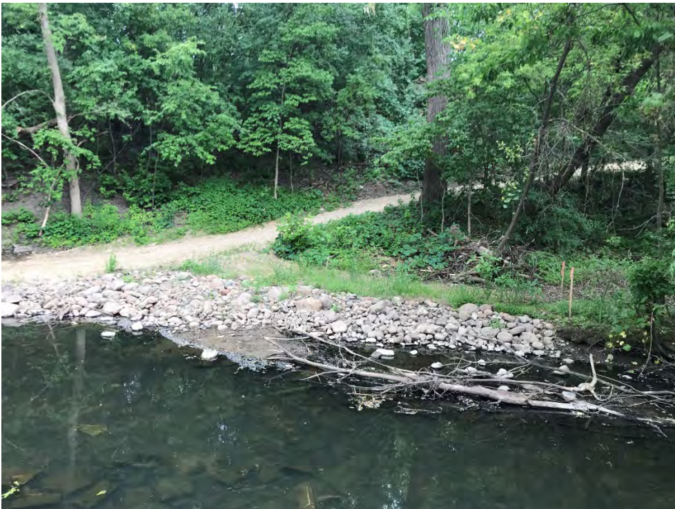
Reach 2: Riprap and native vegetation reestablishment at trailhead from Glenwood Ave. to site (6/17/2021)
