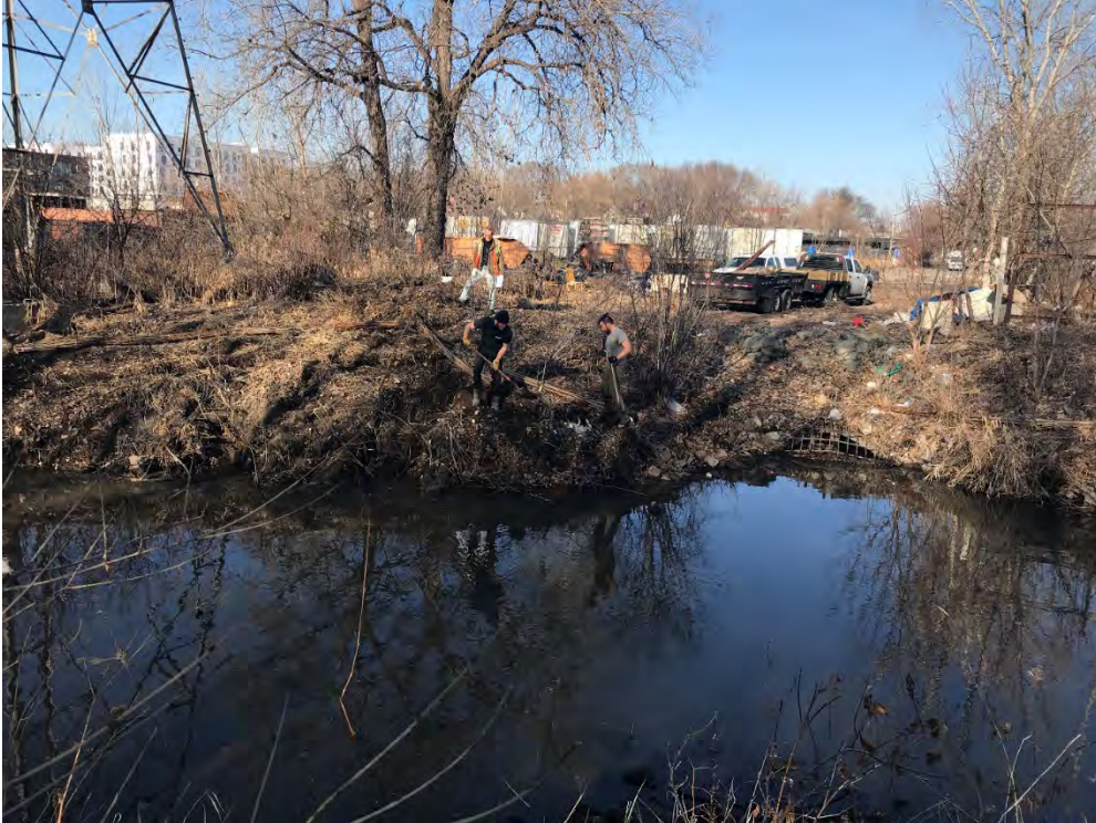
Reach 1: Landbridge Ecological installing fascines near culvert upstream of Van White Memorial Blvd. (12/10/2020)
