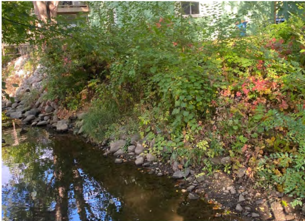
Figure 3: Proposed hybrid armoring technique, as installed in a stream on a previous project
