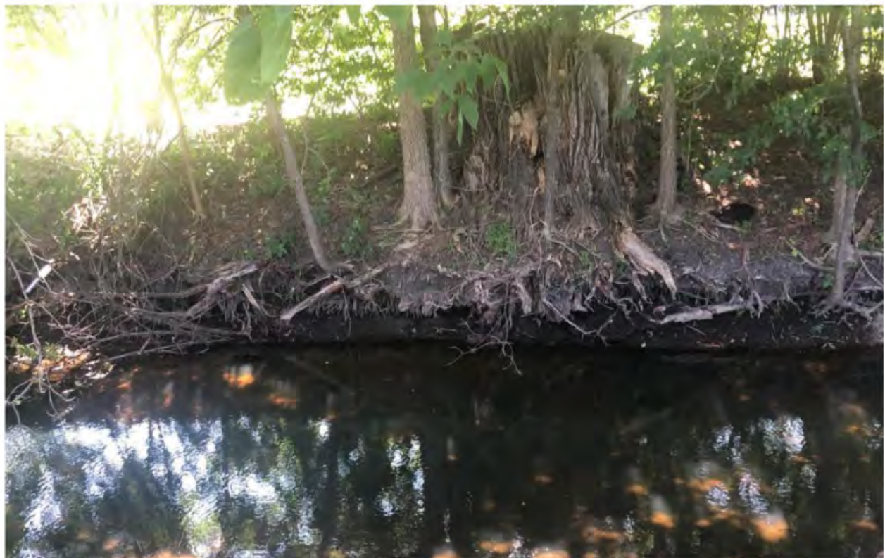
Figure 1: Channel erosion in the proposed project area
