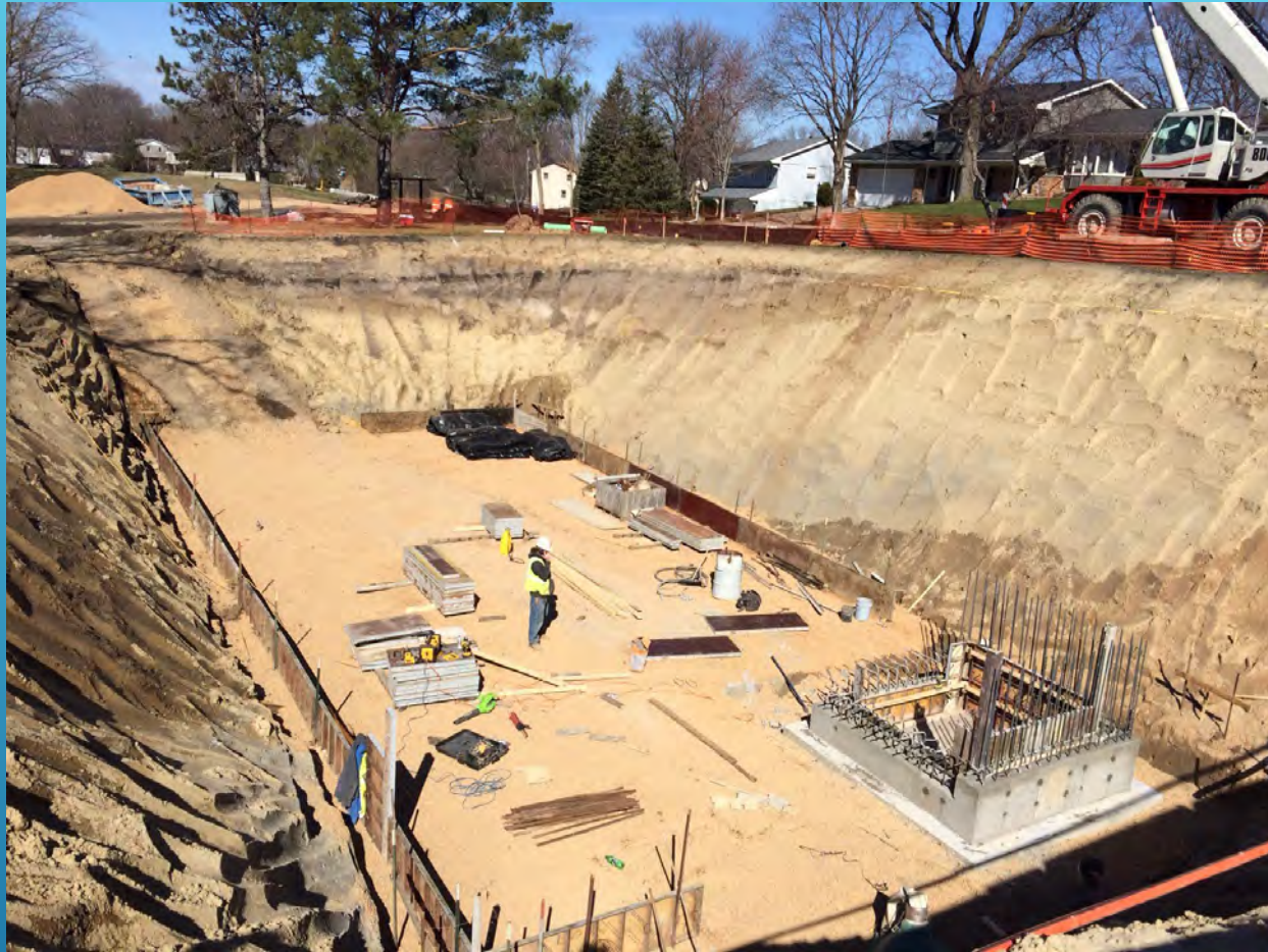
Underground Storage Tank and Adjacent Rain garden
