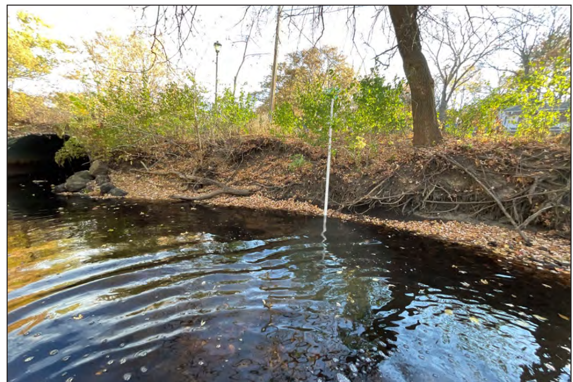
Scour near culverts
