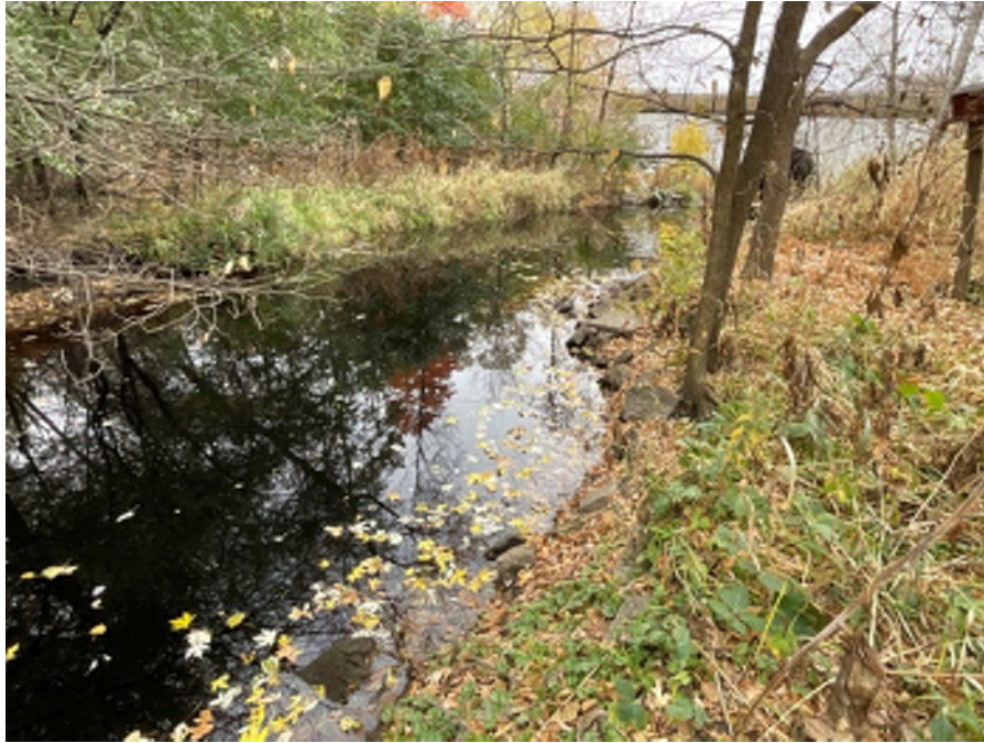
Photo 51: Site 4i. Poor riprap at the right bank of station 70+80 (facing downstream).
