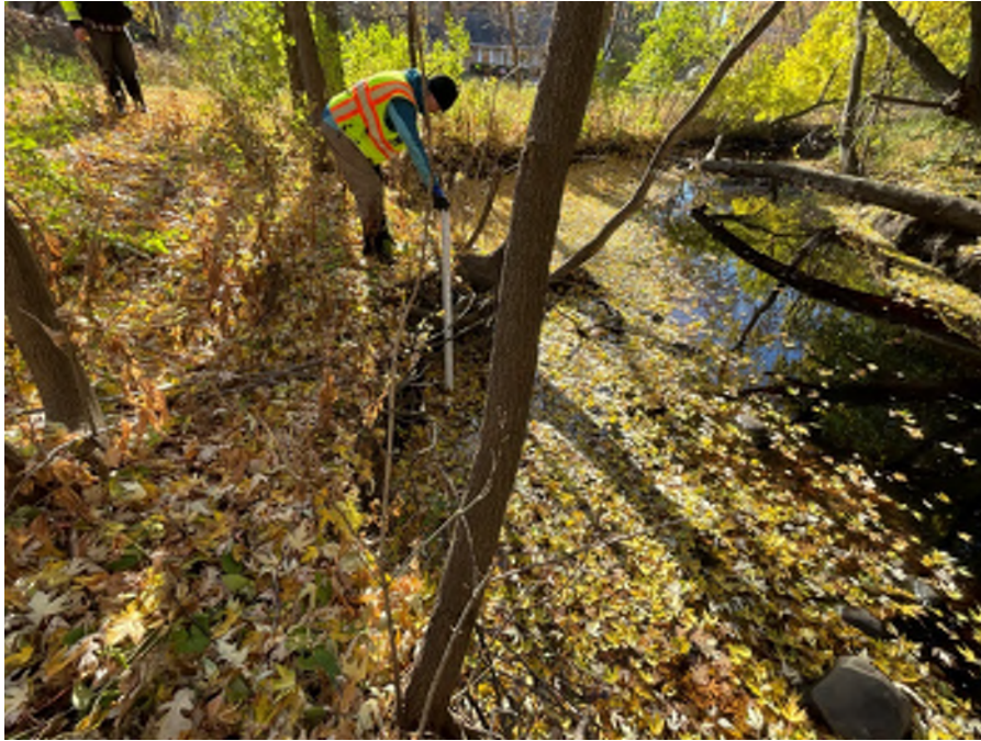
Photo 39: Site 3i. BEHI measurement at the right bank of station 53+00 (facing upstream).
