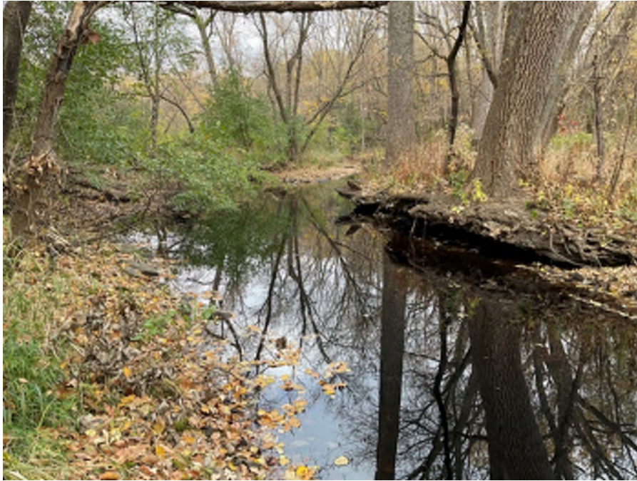
Photo 45: Site 4e. Undercut at station 65+50 (facing upstream).
