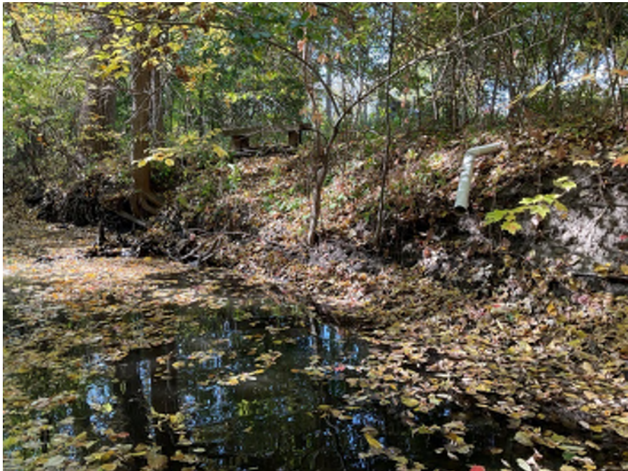
Photo 8: Site 1e. Drainpipe and bare soil on the left bank of station 13+50 (facing upstream).
