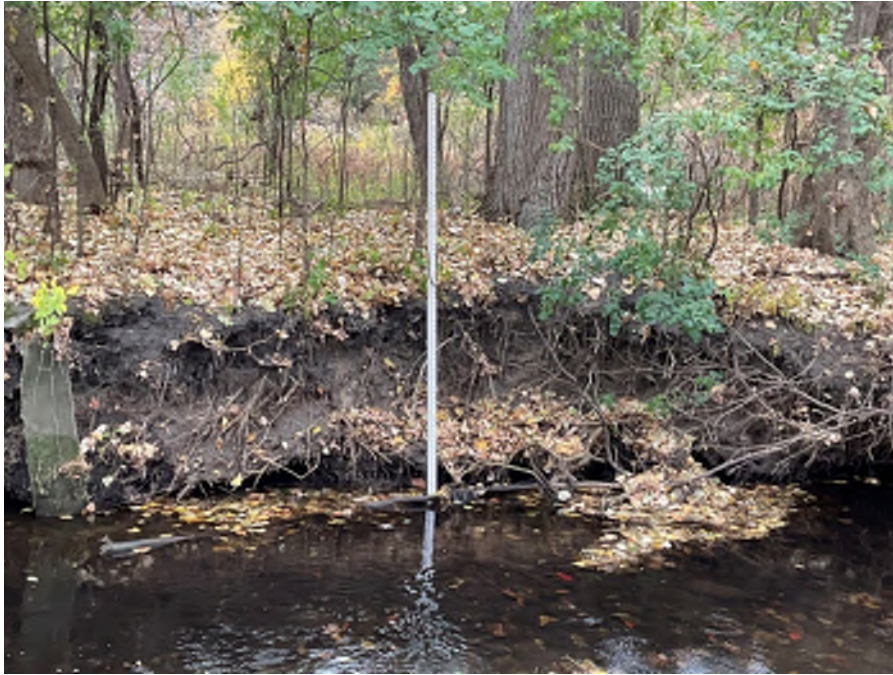
Photo 19: Site 2g. Bare soils and undercutting at the right bank of station 27+60.
