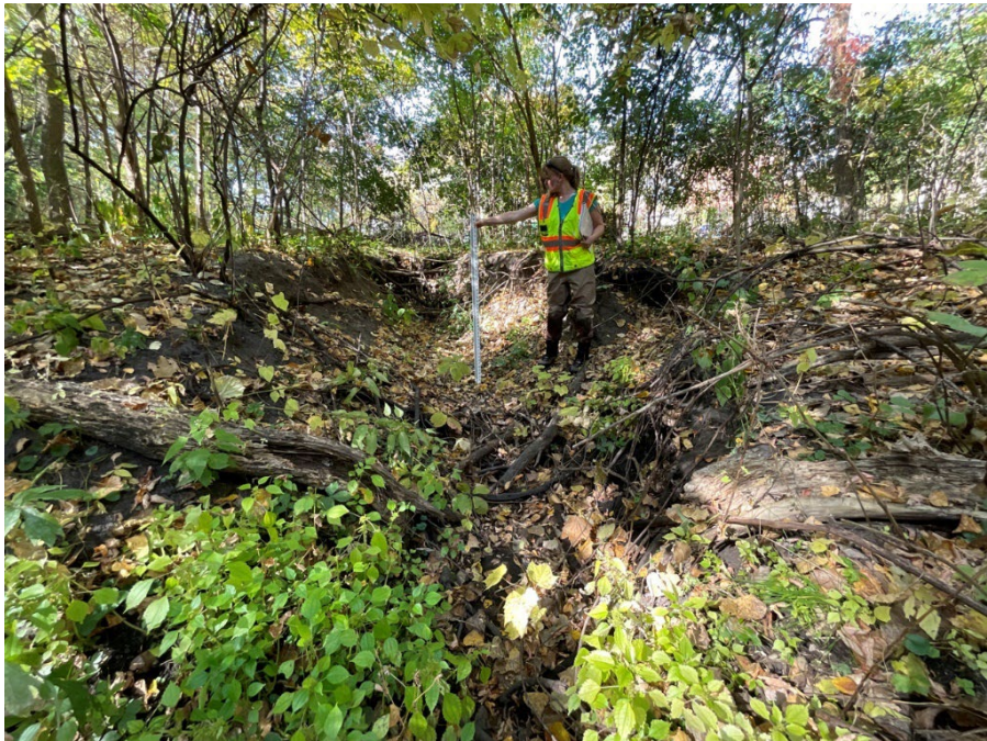
Photo 7: Site 1e. Gully formation from parking lot runoff on the left bank of station 12+20.
