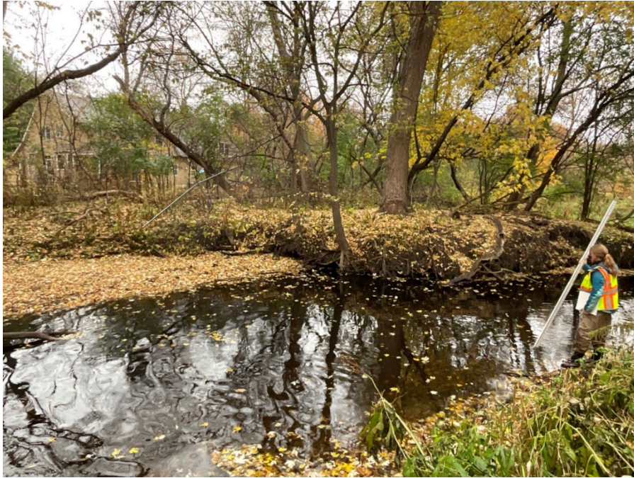
Photo 27: Site 2m. Deposition and undercut at the left bank of station 36+60.
