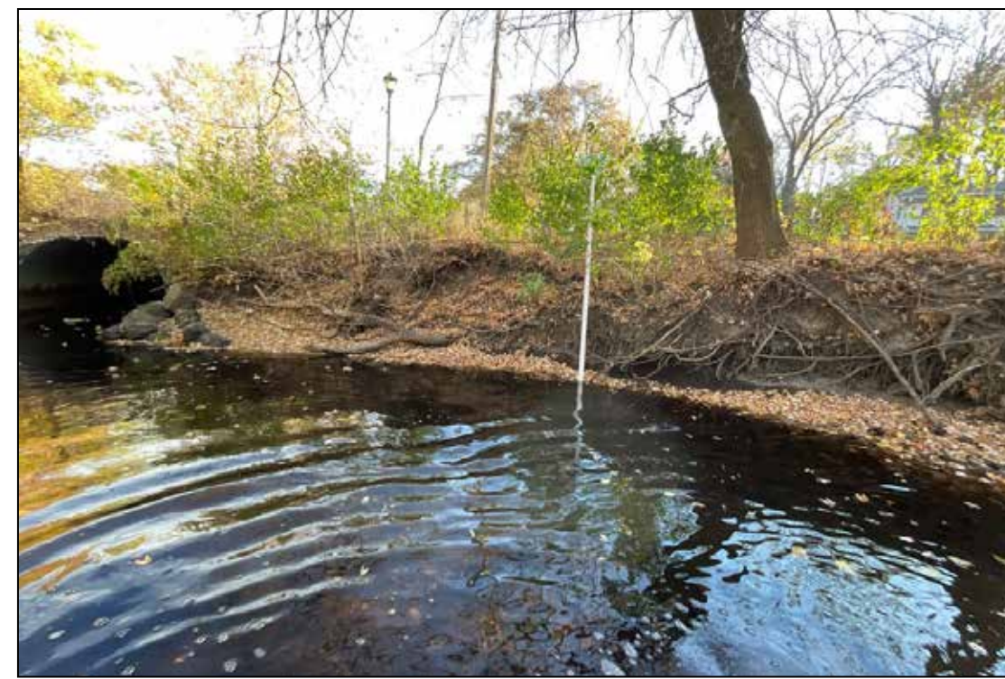
Scour near culverts
