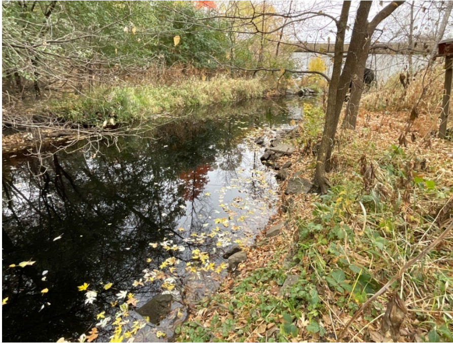
Photo 51: Site 4i. Poor riprap at the right bank of station 70+80 (facing downstream).
