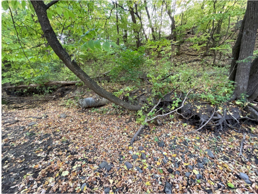
Photo 17: Site 2f. Concrete-filled pipe and right bank undercutting at station 22+75.
