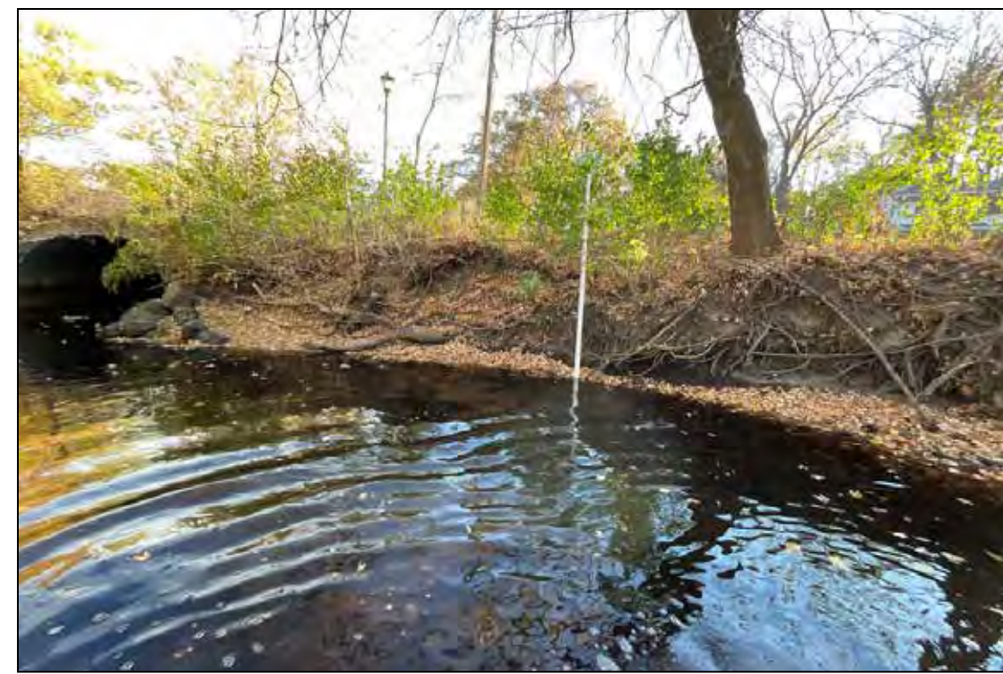
Scour near culverts
