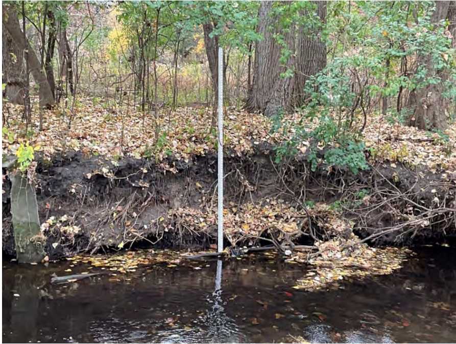
Photo 19: Site 2g. Bare soils and undercutting at the right bank of station 27+60.
