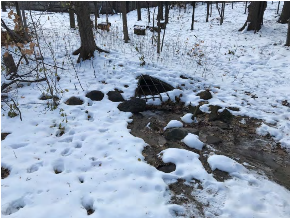
Figure 3-5 Erosion and Sediment Deposition at a Stormwater Side-channel
