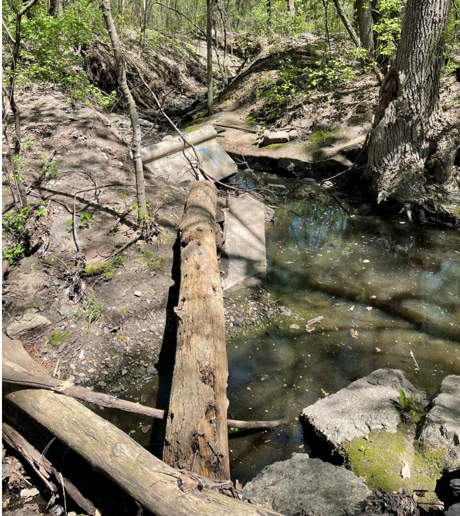
Figure 5-6 Pond SR-4 Downstream Outlet Channel Erosion and Construction Debris
