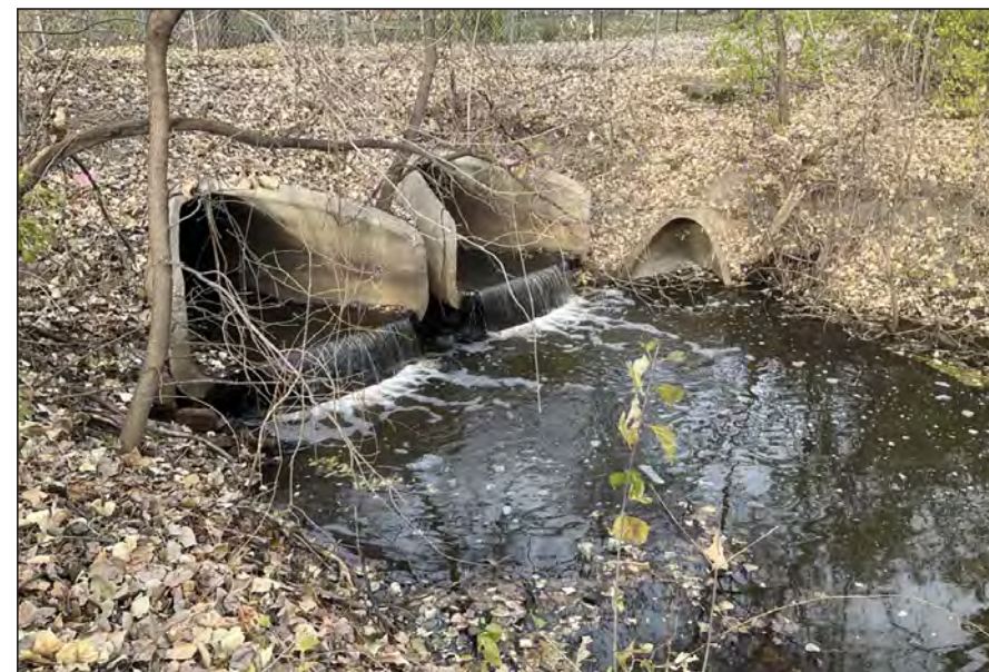
Scour near culverts
