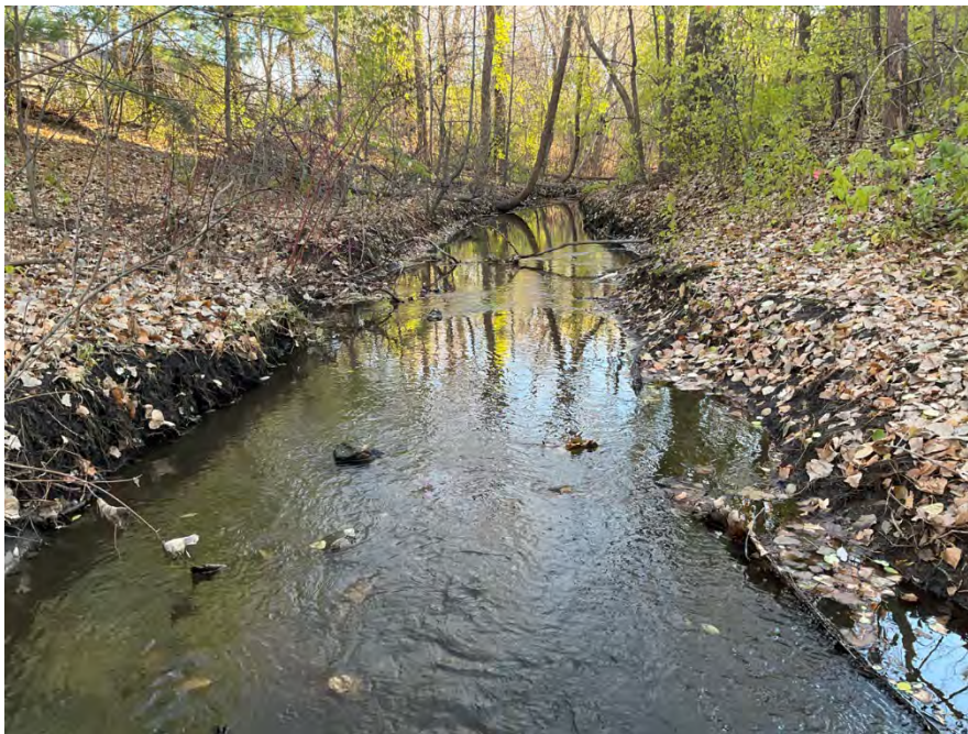
Photo 27: Site 3c. Looking downstream at station 42+90, both banks have minimal vegetative surface protection.
