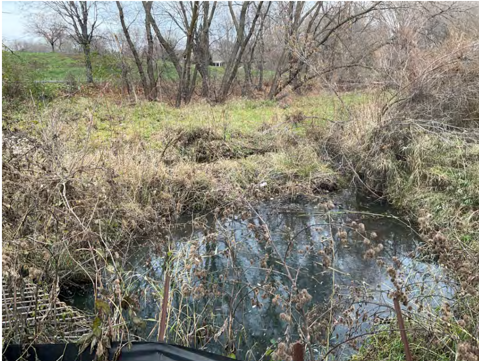
Photo 26: Site 3a. Looking downstream at the sediment island formed at station 37+00 due to the pipe crossing at Vicksburg Road. The island width ranges from 1 to 10 feet wide, is 30-feet long, and roughly 1 foot above the water surface level.
