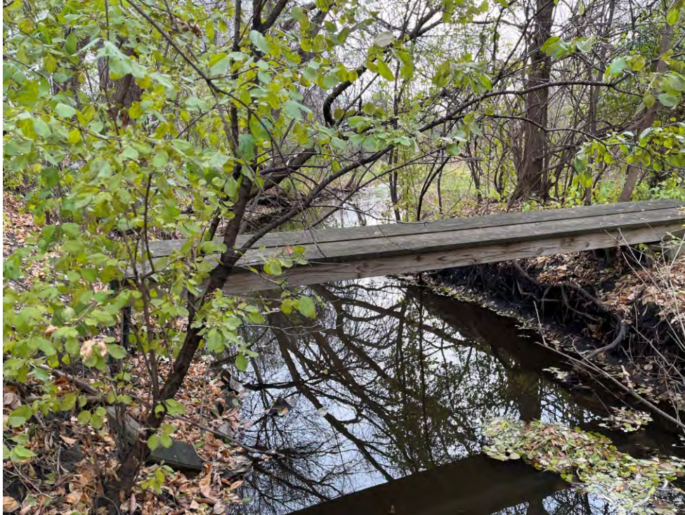
Photo 16: Site 2a. Looking downstream at station 20+30, the right bank is bare and vertical. There are two footbridges in this vicinity.
