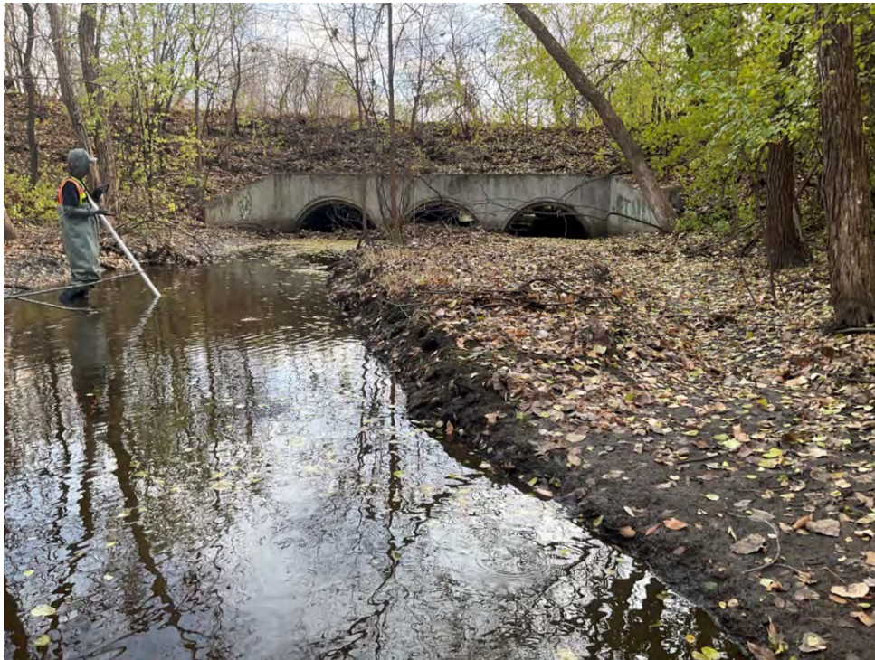
Photo 41: Site 4f. Looking downstream at station 66+90 towards the 38th Avenue crossing. The center and right culvert are partially blocked by sediment deposition.
