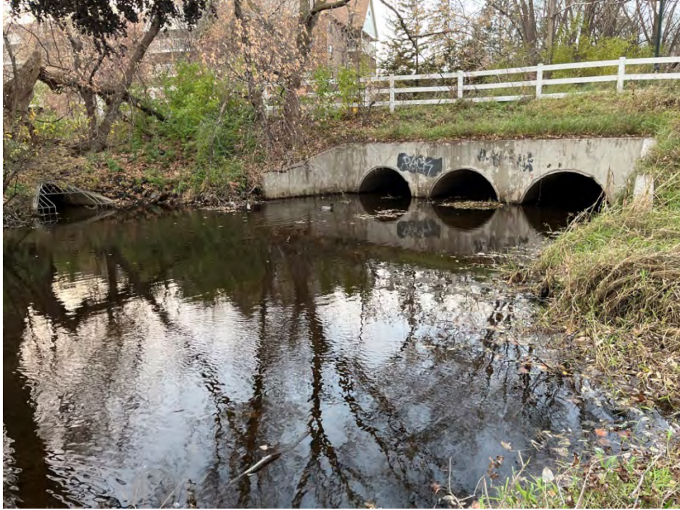
Photo 42: Site 4g. Looking upstream at station 69+00 towards the 38th Avenue crossing. Slight sediment build up in center of channel near the culverts.
