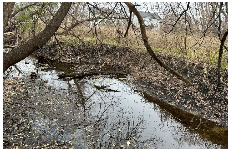
A section of eroding streambank along ǪǪǪ Wakpádaŋ / Main Stem of Bassett Creek evaluated in 2023 (Photo: Barr Engineering Co.).
